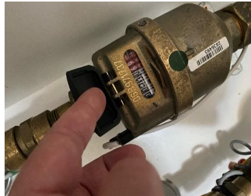
Cold Water Meter Image
